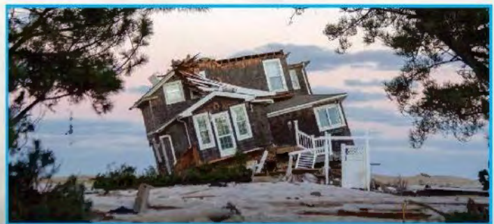
Mantoloking, N.J., Nov. 5, 2012 - This house was destroyed by the storm surge of Hurricane Sandy. FEMA
